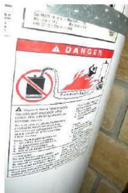
Warning label on gas heated hot water cylinder.
