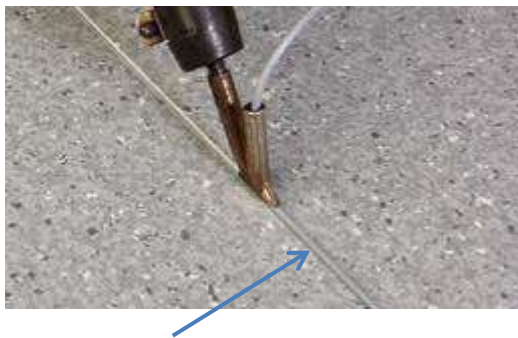
A slight wash of melted weld rod rising at the edge of the weld
