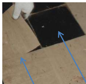
Photo 3 Vinyl asbestos tiles
