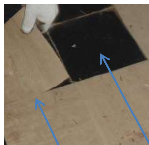
Photo 3 Vinyl asbestos tiles Bitumen adhesive with asbestos fibres
